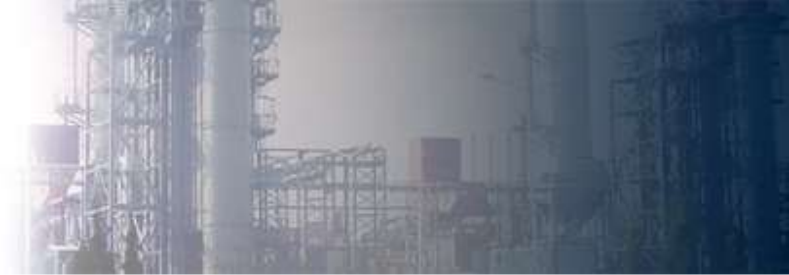
Ankara Natural Gas Combined Cycle Power Plant Ankara / Turkey / 2001 Client : Va-Tech - Yüksel Construction Co. Consortium.
